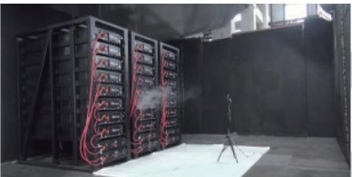
(e) Thermal runaway in Cell 36
